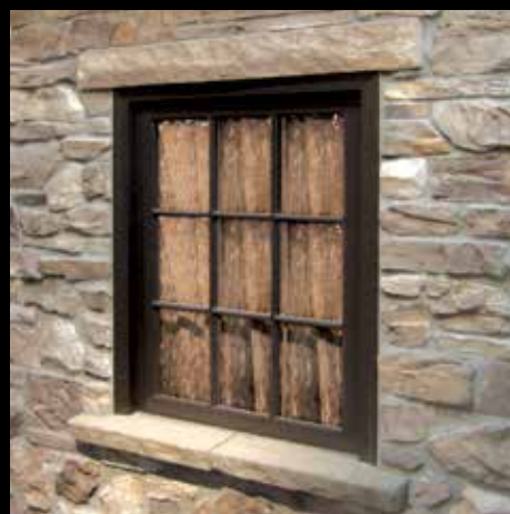
Chiseled Stone Lintel - Volterra (Above Window) Split Stone Sill - Volterra (Below Window)
