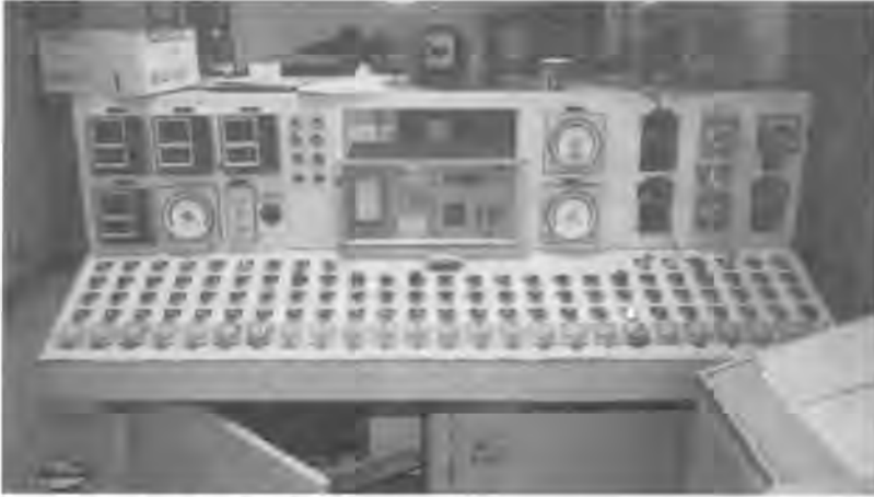
Console at the Ouachita plant that controls temperature and monitors functions in the tunnel kilns.
