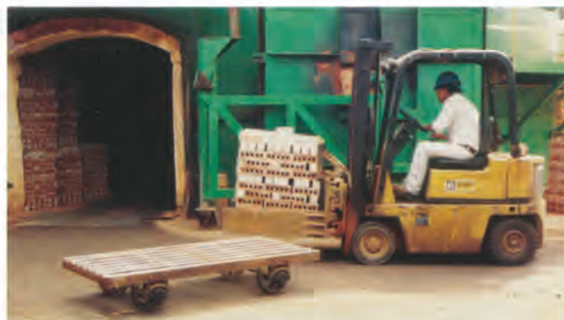
Filling a thin clad kiln at Bridgeport with dried brick prepared for burning.
