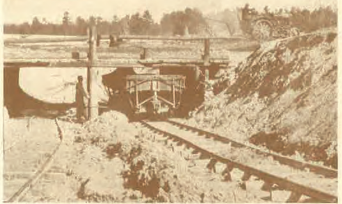
Loading the Clay on Cars for Delivery To the Clay Storage Building
