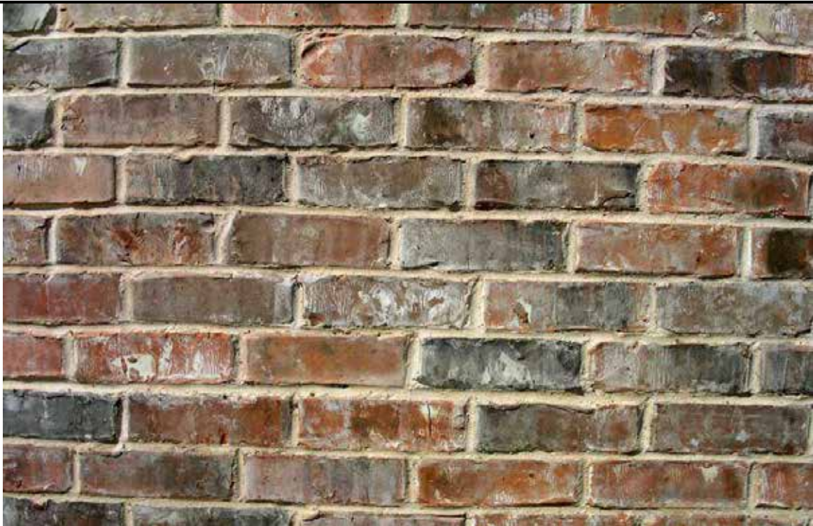
Figure 1. Brickwork with dryer cracks viewed five feet away. At twenty feet they are not visible.
