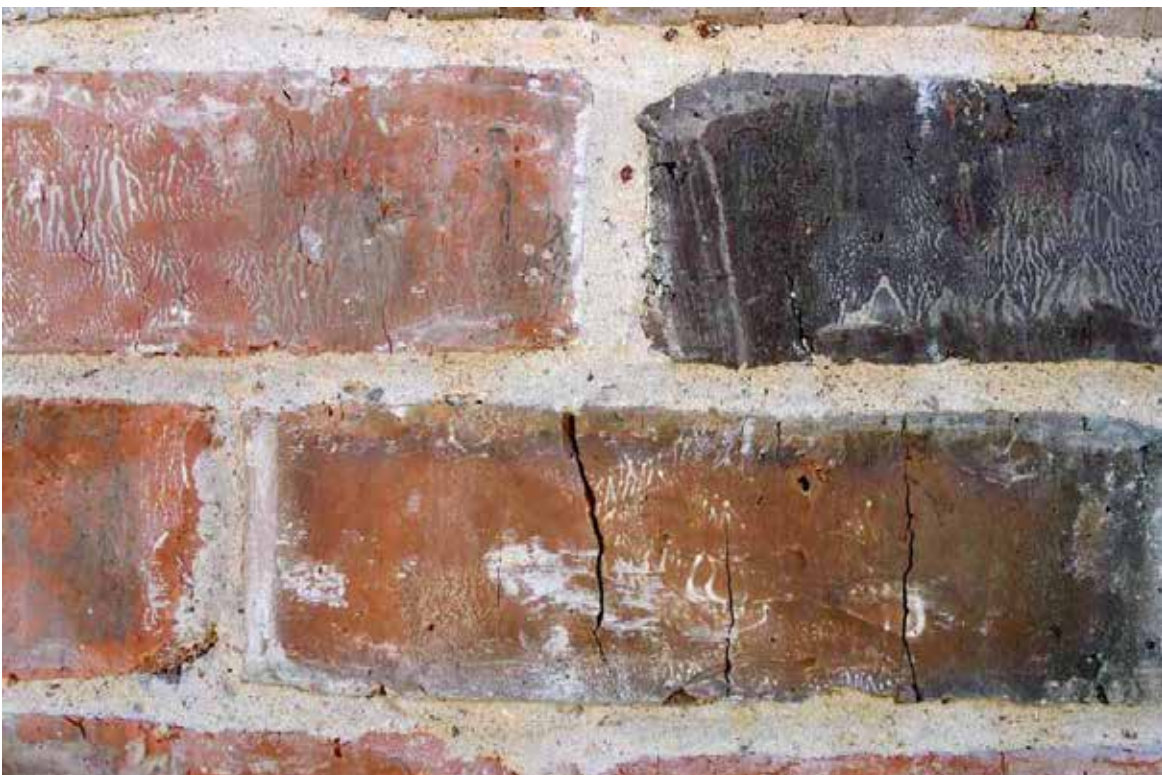
Figure 2. Close-up of a brick in that wall with dryer cracks.
