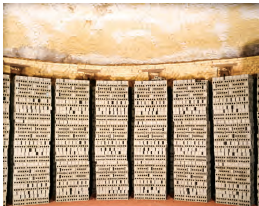
The interior of a beehive kiln, a completely self-supporting structure, is captured in these images.
